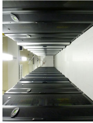
Hardware1: TSUBAME2 supercomputer
